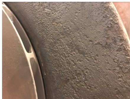
Figure 4.1: Fouled last stage diffuser hub of retired multistage compressor previously operating at Åsgard - now located at the NTNU wet gas compression facility.
