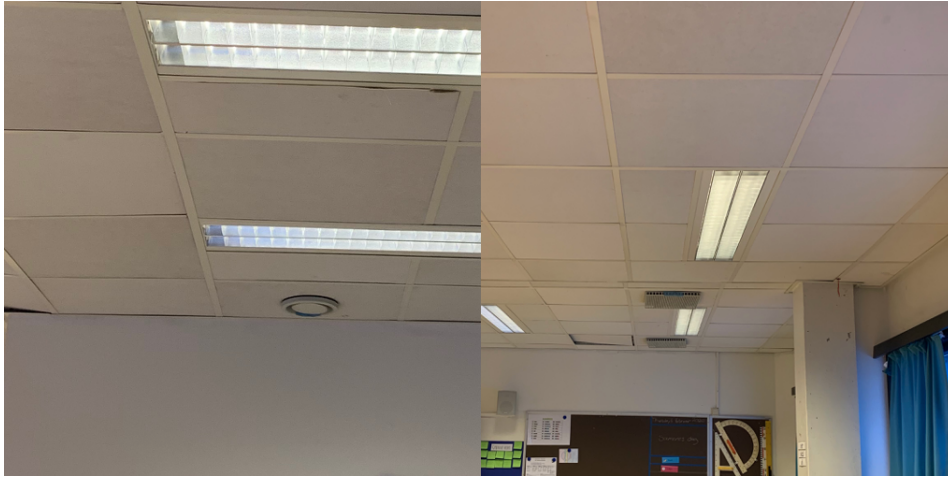
Figure 4.2: An example of the ventilation distribution system at Stabbursmoen school. A typical extract is seen left in the picture and a typical air supply grill is seen to the right
