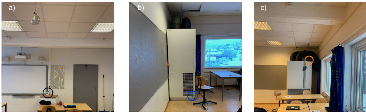
Figure 3.9: Location of placement of sensors in classroom 104. a) Sensor, measuring air quality b) Sensor measuring temperature of supply-air, and c) Sensor measuring temperature of extract-air
