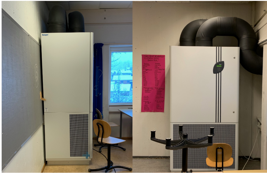
Figure 4.4: An example of a classroom ventilation aggregate from Swegon. This type of ventilation unit supplies to four classrooms at Sunnland school
