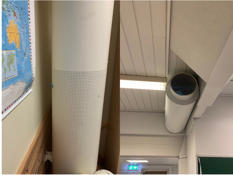
Figure 4.6: An example of the displacement ventilation distribution system at Sørborgen school. A typical extract is seen left in the picture and a typical air supply grill is seen to the right
