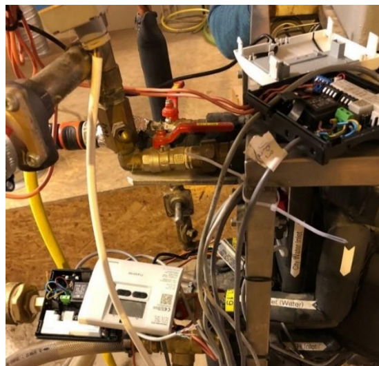
Figure 4.13: The two MULTICAL 403 energy meters during mounting
