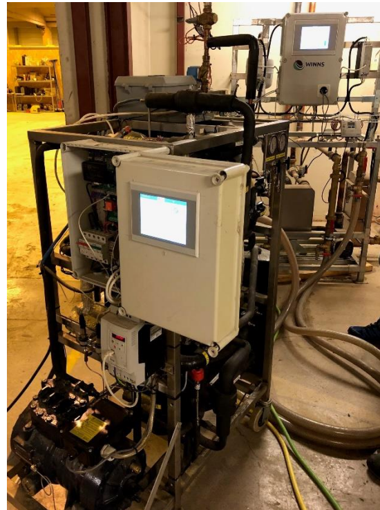
Figure 4.9: The heat pump in the test rig during initial testing
