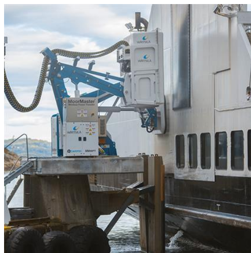
Figure 35 Induction charging solution for ferries (Wartsila 2018b)
