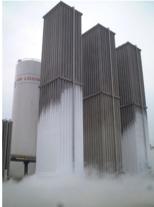
Figure 27 Frost on air-based vaporizer tower (Cryoquip)
