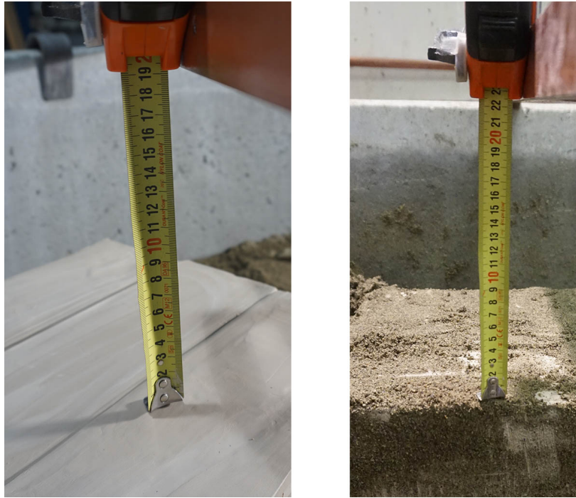
Figure A.50. Local depth of the top of clay layer. Left: When constructed. Right: When excavated.
