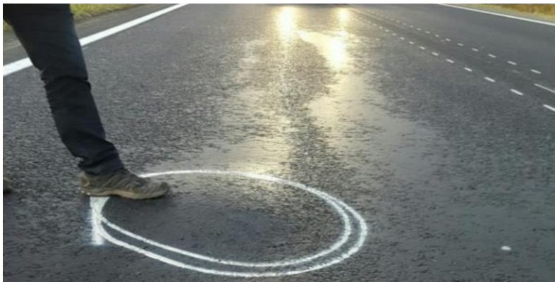
Figure 1: Blister in a Norwegian asphalt pavement road (Hovin, 2018)
