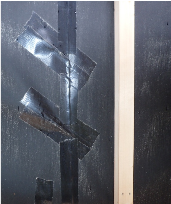
Figure 1: A taped joint in the wind barrier of the ZEB Laboratory. Tape is also used to repair minor tears in the wind barrier.
