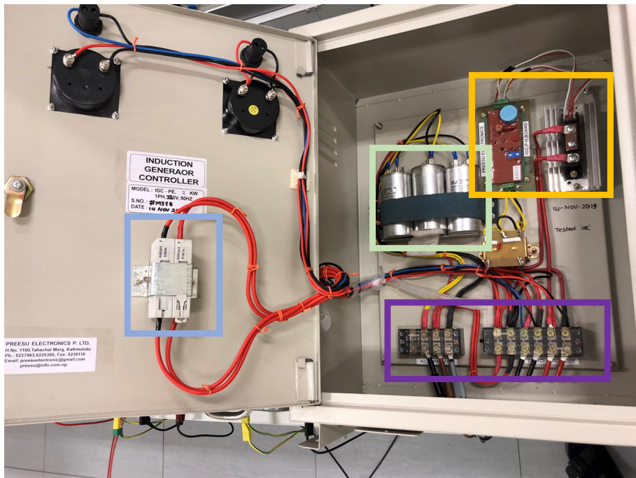
Figure 2.23: Picture of the inside of the electric load controller, showing the connection ports to the generator, the ballast load and village load in the purple box. The capacitors are shown in the green box, the thyristor and main board are shown in the yellow box, and the backside of the switch are shown in the blue box below two voltage measurement are at the door
