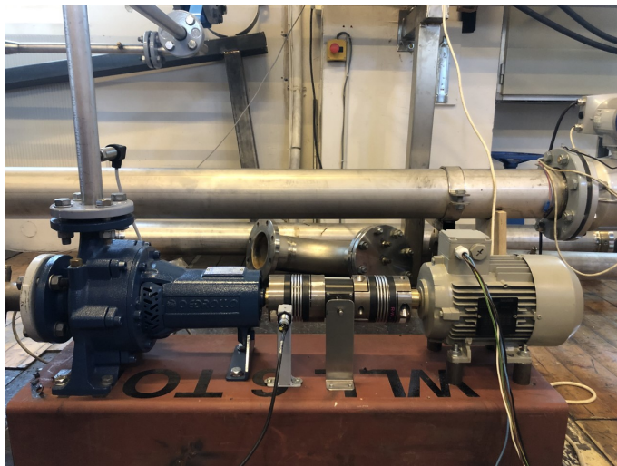
Figure 6.2: Picture of the direct connection of the PAT (to the left) and the induction generator (to the right)
