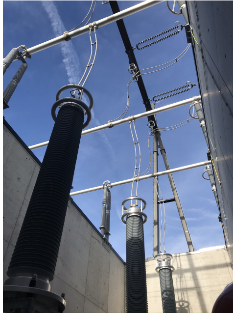
Figure 7.2: Transition between the overhead power lines and the cables that are entering the culverts.
