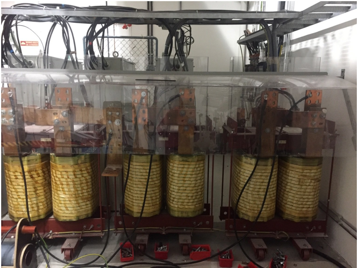
Figure 3.4: The transformers used as an energy source.
