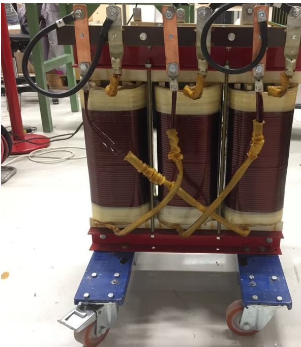
(a) The primary side of the test transformer.
