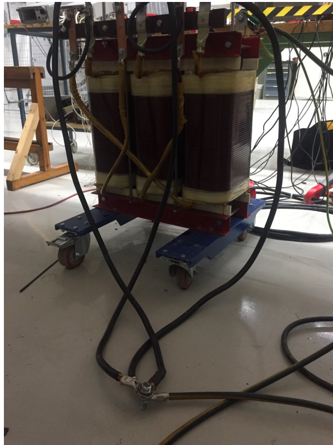
Figure 3.2: Short circuiting of the primary side of the test transformer.
