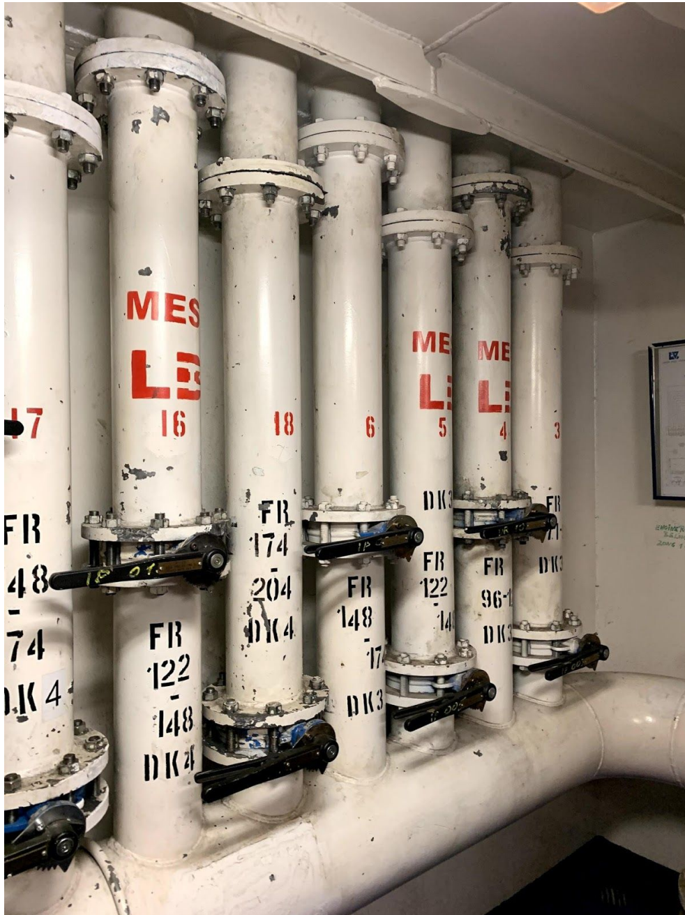
An image of the drencher room. Pictured is the manual valves that open the flow of water to a drencher section. Next to the valves is a phone that should be used to inform the bridge of which drencher section has been activated. The pipes are marked with drencher section numbers, which beam it includes and whether the section contains lifeboats.
