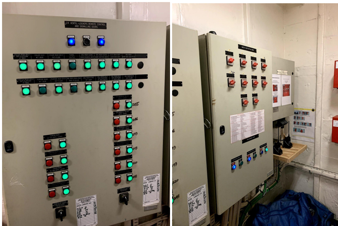
Two images from the safety station. This station also functioned as a fire station. Here you can activate the ventilation safety stop, close fire doors remotely and shut off the fuel supply to the engine.
