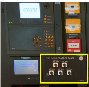
Figure 2.23 Bridge remote control of fire doors (marked in yellow) on MS Newbuilt Explorer . The doors are configured to automatically close in the event of a fire alarm. The crew can remotely close all fire doors in a specific main vertical fire zone, or all fire doors onboard.
