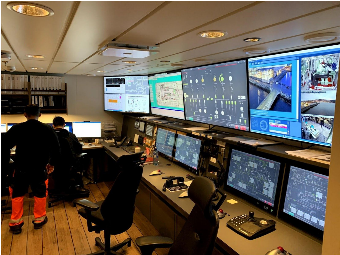
Image from the control room. This room is next to the engine room and contain control systems for the engines. In addition, a fire station is installed here, as well as CCTV access panel.
