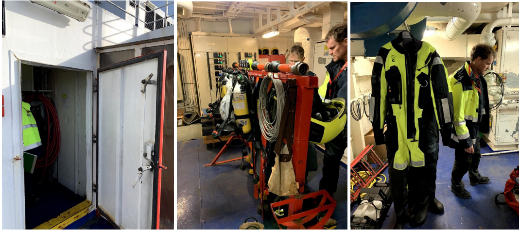
Images from fire station #3. This is where the chief engineer and fireteam muster in the case of a fire. The room contains fire equipment and smoke diver equipment.
