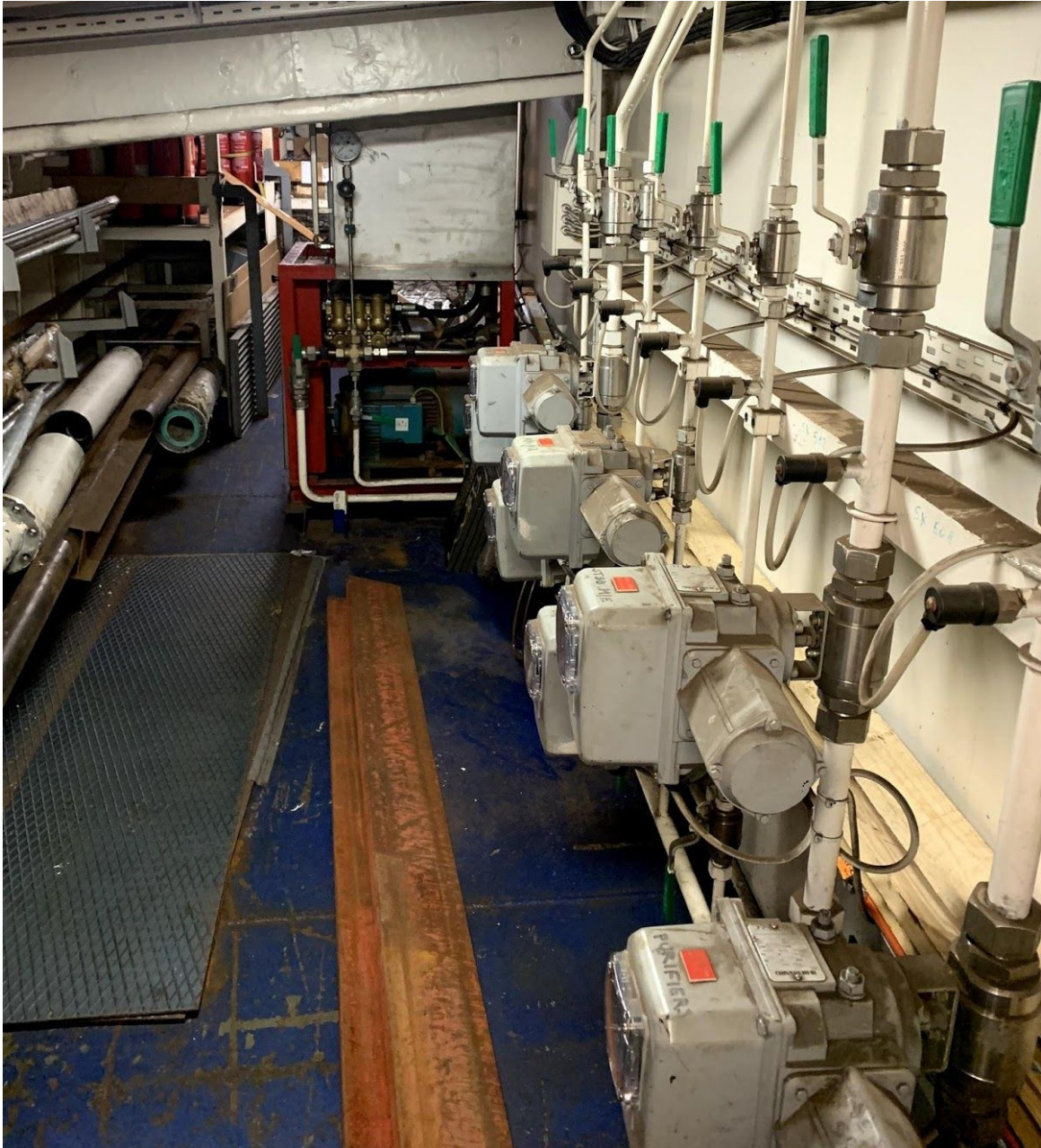
The HiFog pump room. The different HiFog zones can be started manually from here, but they can also be started remotely from the bridge.
