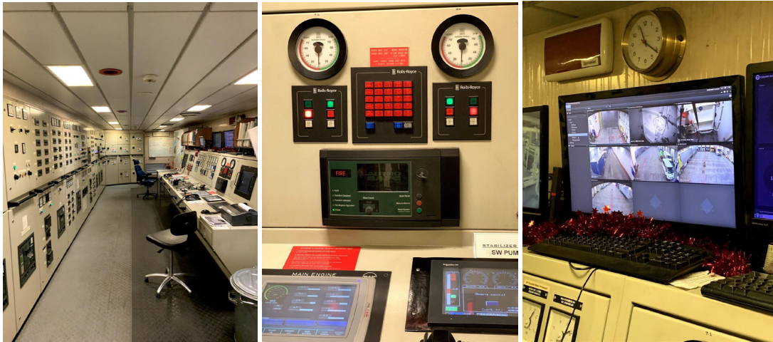
Images from the control room. A separate CCTV system and a fire detection panel are located here.
