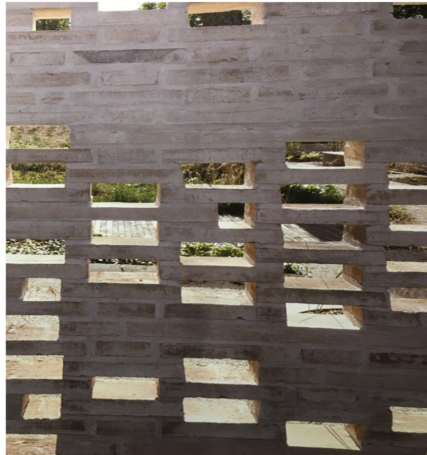
Fig. 21. Detail of the sheltering brick wall that wraps the perimeter of the center. Glazed Danish bricks of varying sizes and view openings create a sense of shelter while allowing glimpses of the surrounding community and landscape.
