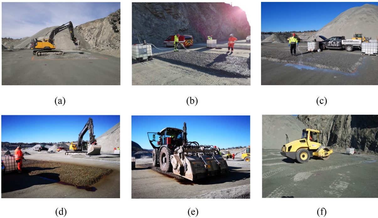
Fig. 4. Construction of the first 15-cm course of the base layer: laying of the material (a), spreading water at L0 (b), spreading polymer-based additive at L1 (c), spreading lignin-based additive at L2 (d), mixing (e) and compacting (f).
