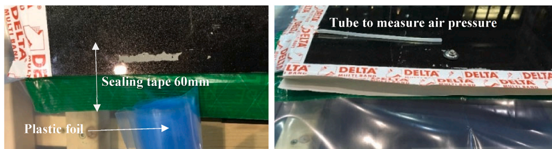
Fig. 5. Sealing the edges of the BIPV system using sealing tapes and polyethylene foil (view from the frontside). On the right photo a tube used to measure the differential air pressure is visible lying on the black module. Study 3 (Table 3).
