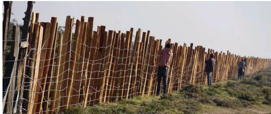
Fig. 1. Fences under construction in Pardamat village in the Maasai Mara (Photo: Author, 16 October 2017).
