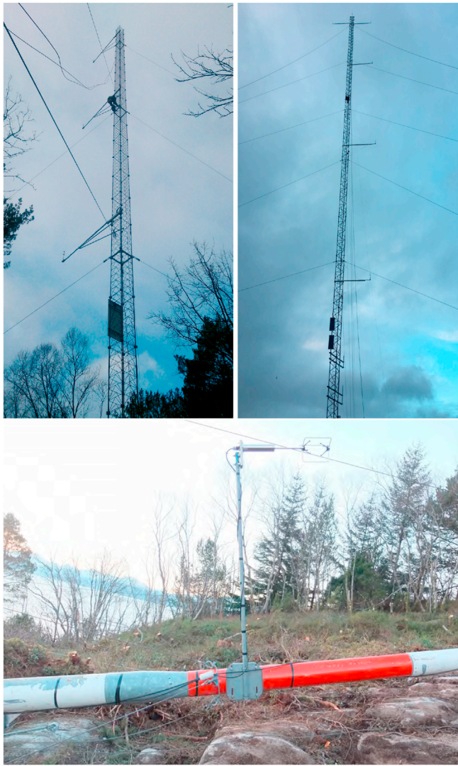
Fig. 4. Examples of mast structures used. Rectangular lattice tower at Aakvik in Halsafjorden (upper left), Kvitneset in Sulafjorden (upper right), and Halsanaset in Halsafjorden (below), where one of the anemometers can also be seen. Photos: Kjeller Vindteknikk.
