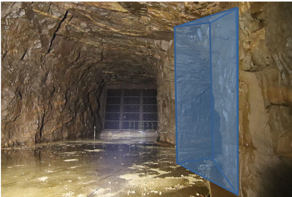
Figure 137: Suggestion of concrete wall wedge to keep the flow patten equally to improve sedimentation
