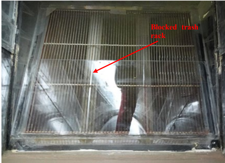
Figure 46: An overview of the weir height at trash rack after modification 2
