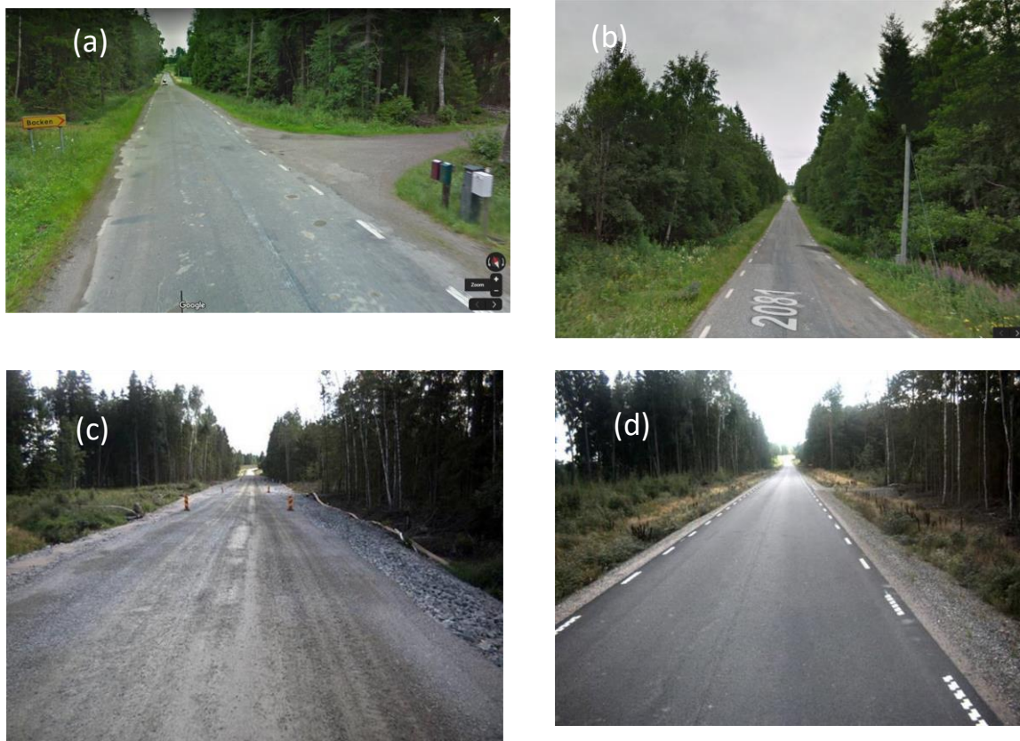
FIGURE 1. Pictures of study area, (a) prior to upgrading July 2011 (from Google maps), (b) during the ground investigation works by Skanska in Summer 2015, (c) during the upgrading works in Spring 2016 and (d) after completion of the works in August 2018. Photographs from pmsv3.trafikverket.se
