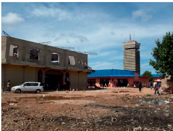
Chinese owned shops under construction, between Kamwala Market and the intercity bus station.
