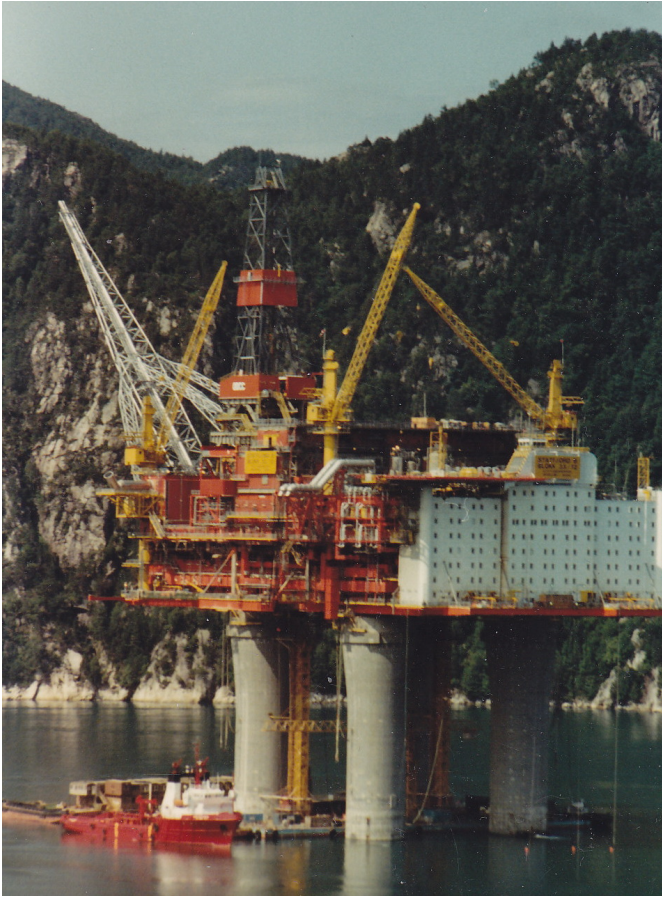
Figure 1.1: The Condeep platform Statfjord B during construction in Vats, Norway, 1981. Photo: Jon Natskår.
