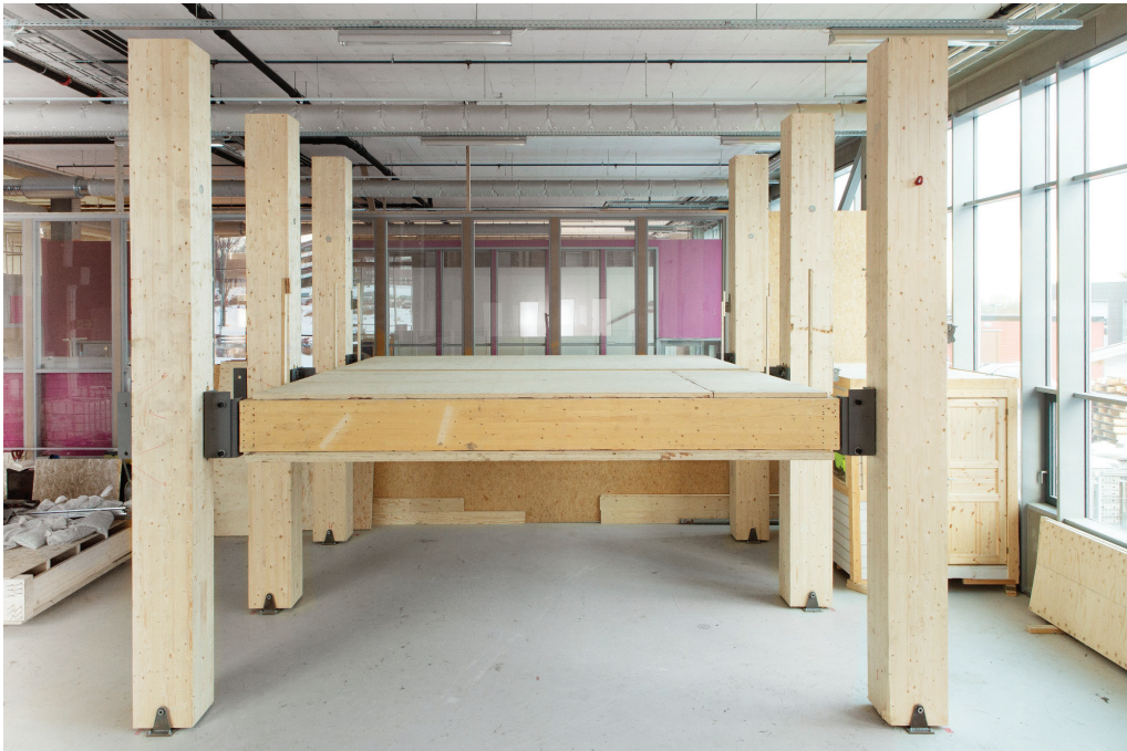
Figure 1 – Woodsol prototype installed at Charlottenlund Videregående Skole, Trondheim (Norway)
