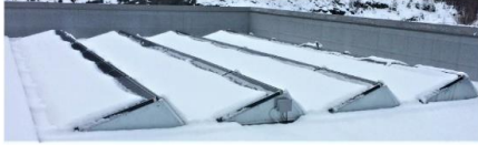
Fig. 3. Photo of snow covered PV installation on a roof near Trondheim, Norway. Snow can be seen to have begun to slide but has been hindered due to build-up. Courtesy of GETEK Energy AS (Norway).
