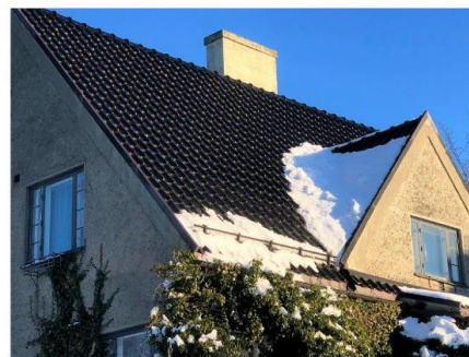
Fig. 2. Snow guard. Photo of a snow guard holding snow on a residential roof in Trondheim, Norway.
