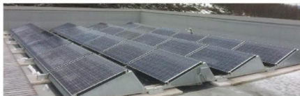
Fig. 1. Photo of frost accretion on common PV installation on a roof near Trondheim, Norway. Courtesy of GETEK Energy AS (Norway).
