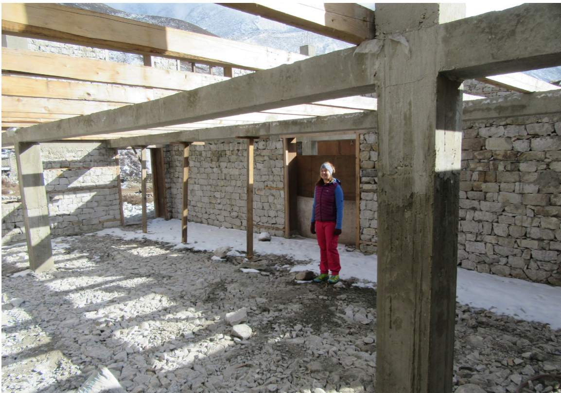
Inside the construction, visible sagging of concrete beams
