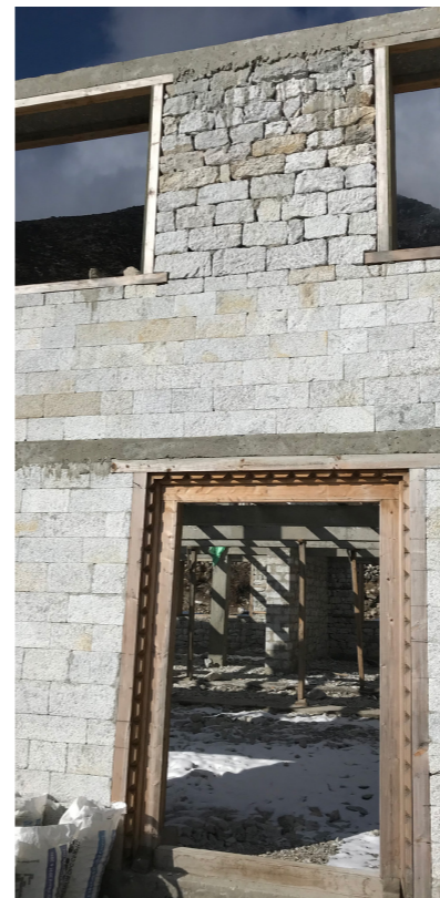
Varying quality of stonework, wooden door and window frames
