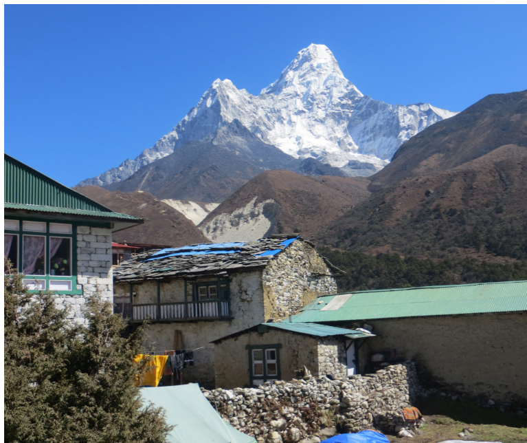
The Yak herders house - patched gable that collapsed in the 2015 earthquake
