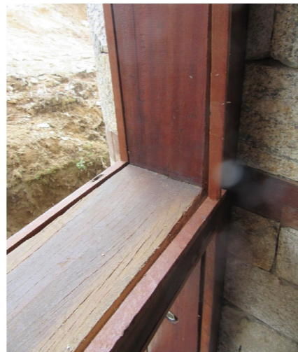
Water damaged window
