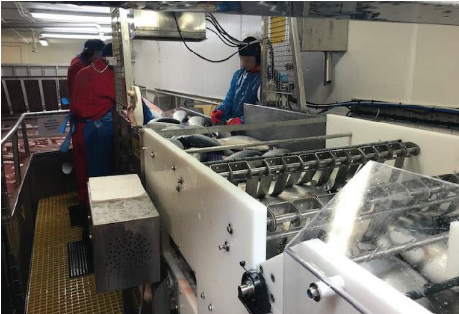
Figure A.12 Slaughter line at FPP 7. Notice the much lower ceiling height at this facility compared to other facilities.
