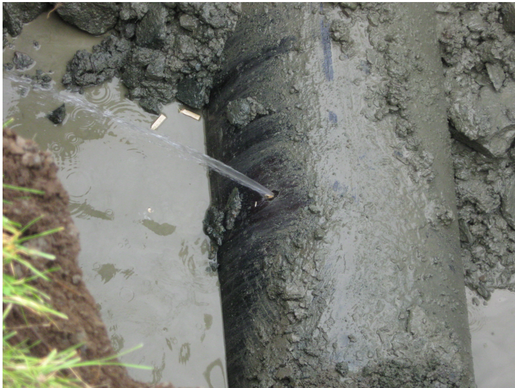
Figure 1.3: A Typical Leak
