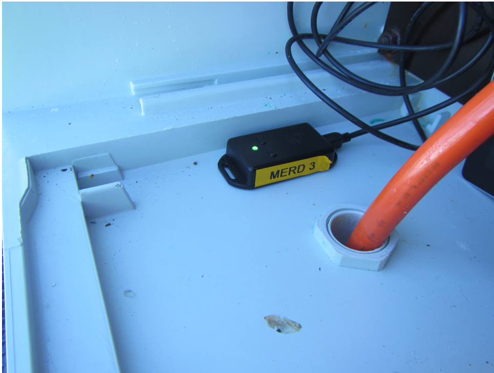
Figure 4.2.6: Image of the alignment of the IMU's inside the power cabinet. Source: Stemsrud (2018)
