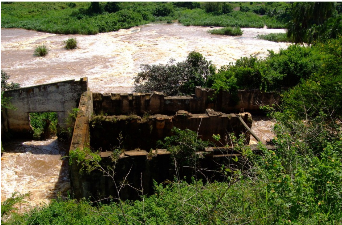
Figure 3. Project site. Remainings of the old Kikagati Power Station seen from the Ugandan side.
