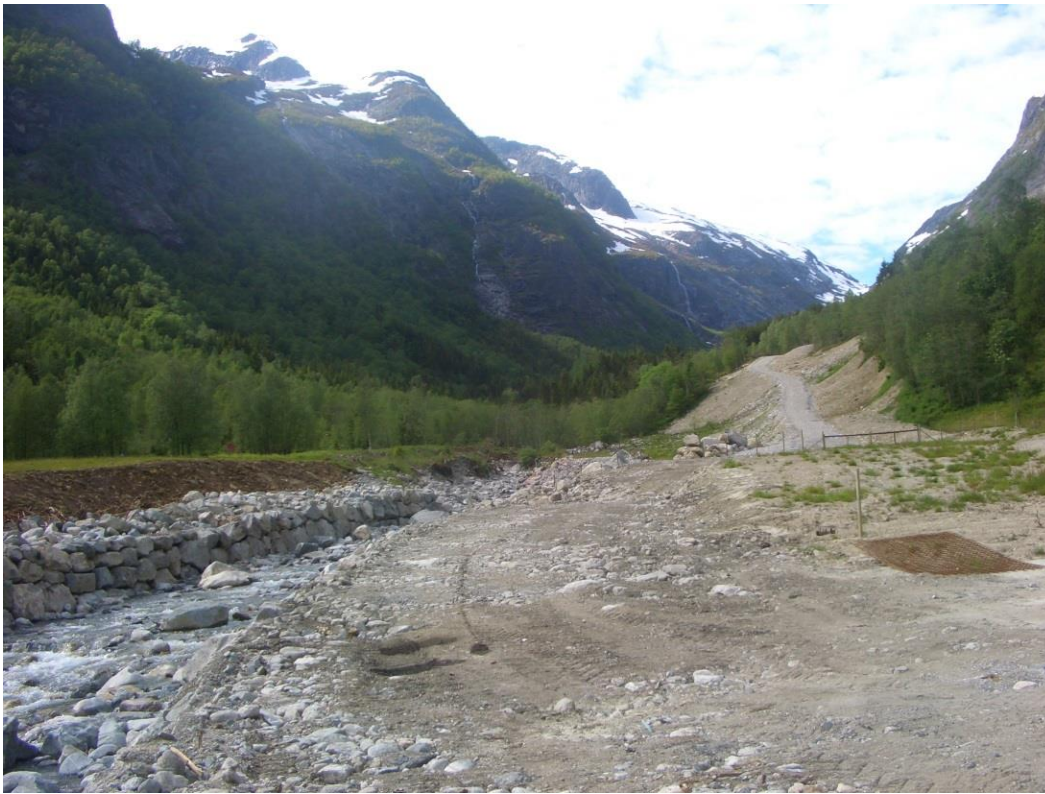
Figure 3.3: Area directly affected at Sværen small-scale hydropower plant. Source: Tor Haakon Bakken.
