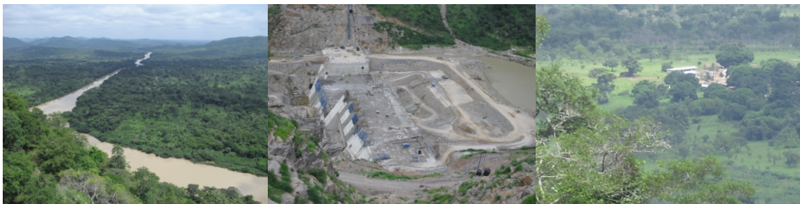
Figure 5: From left, the Black Volta River flowing through the forest at the Bui gorge, the Bui dam under construction and the Bui village preparing to be resettled
