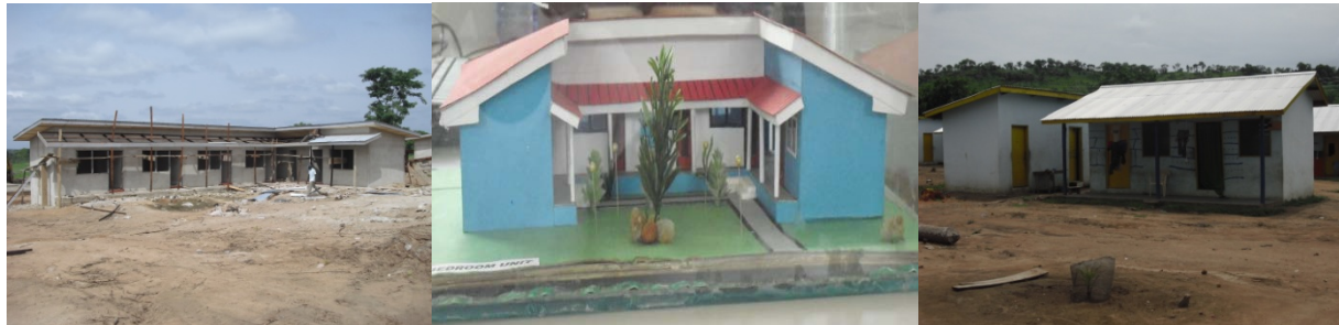
Figure 7: From left a house under construction for phase ‘B’ at Bui, next a model of the house planned to be constructed and the third is a two room apartment with detached kitchen and bath at Gyama settlement
