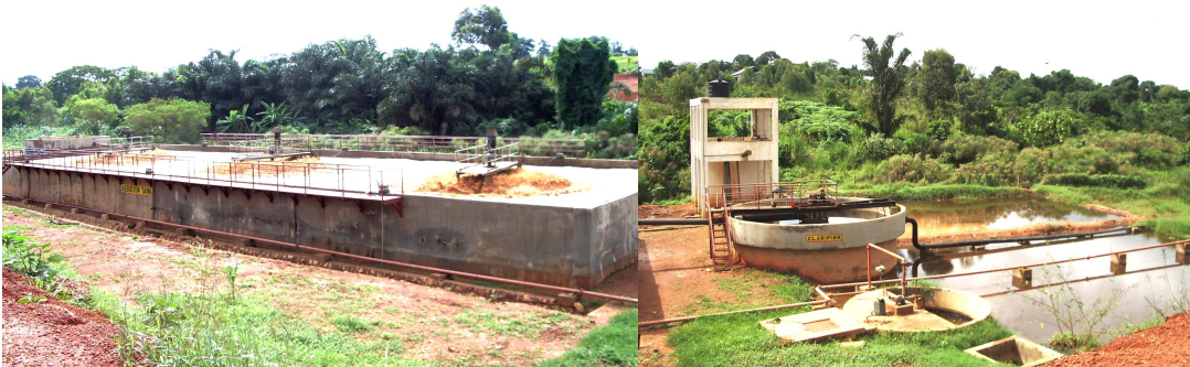
The bio treatment tank
