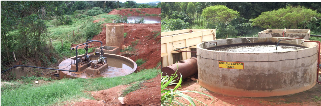
The sump/collection tank
