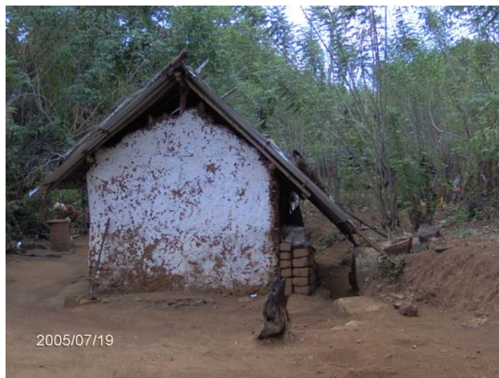
Picture 6.5. Condition of a House in the Study Area
