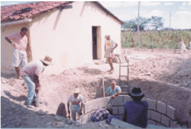
Figure 16: Construction of a rural cistern of the P1MC in the Northeast region. Source: ASA
