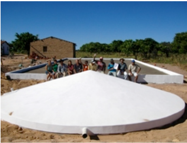
Figure 19: One of the cisterns for food production constructed by the program P1+2 in the community of Girimun in the municipality of Pio IX in the state of Piauí. Source: ASA
