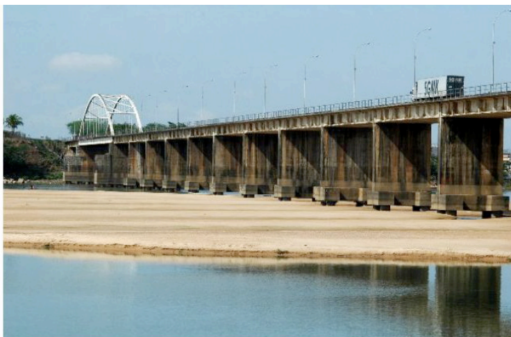
Figure 15: Region of the Low São Francisco river in the municipality of Propriá, state of Sergipe where the reduced levels of the river can be seen in the bridge. Photo: João Zinclair.
