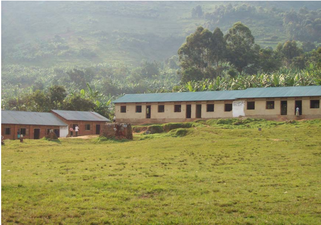
Plate 3 A new five classroom block under construction at Mukono primary school that was funded by an American tourist.
