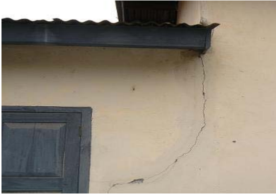
Fig 6 Picture showing cracks in building Source: photo taken by author (July 2006)
