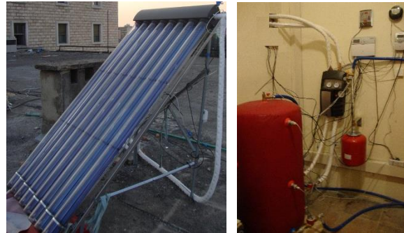
Figure 1. View of the external and the internal part of the solar water heating system
