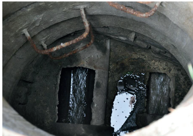
Figure 1.4 Combined manhole can be a source of unwanted water I/I in separate sewers.
