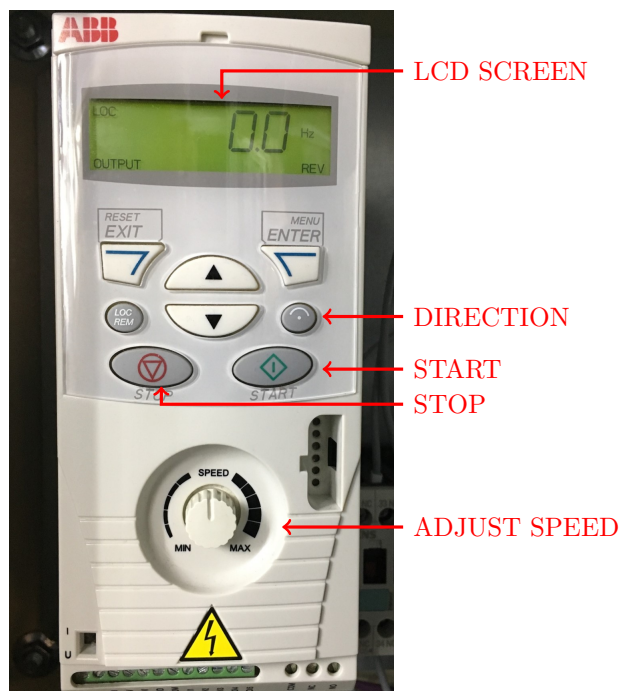
Figure 4.3: Control panel for the mechanical pump.
