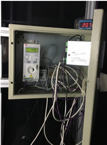
(b) Control panel for the pump
