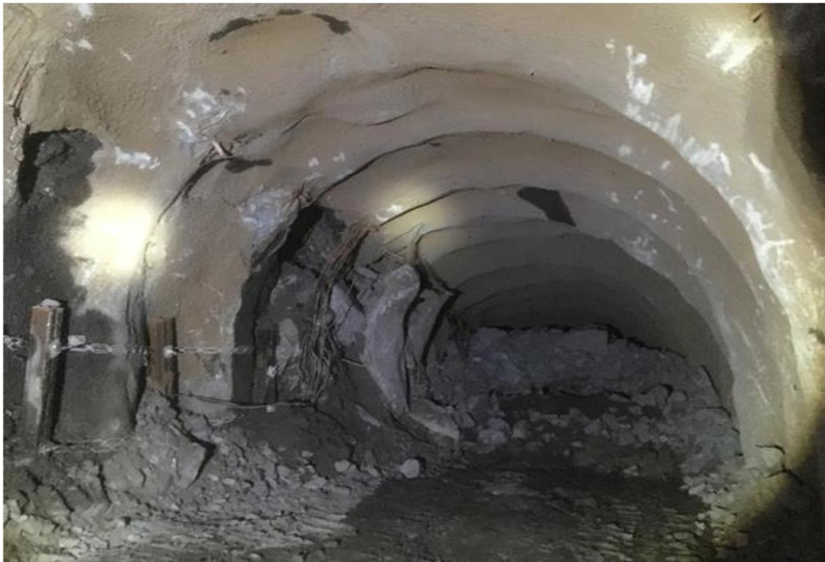
Figure 3. Failure of the reinforced ribs of sprayed concrete and slide in the Matre Haugsdal tunnel in 2017 Brende et al. (2018).
