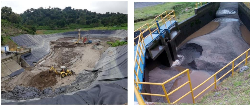
(a) Sedimentation in peaking pond (b) sediment deposited in settling basin during heavy rain
