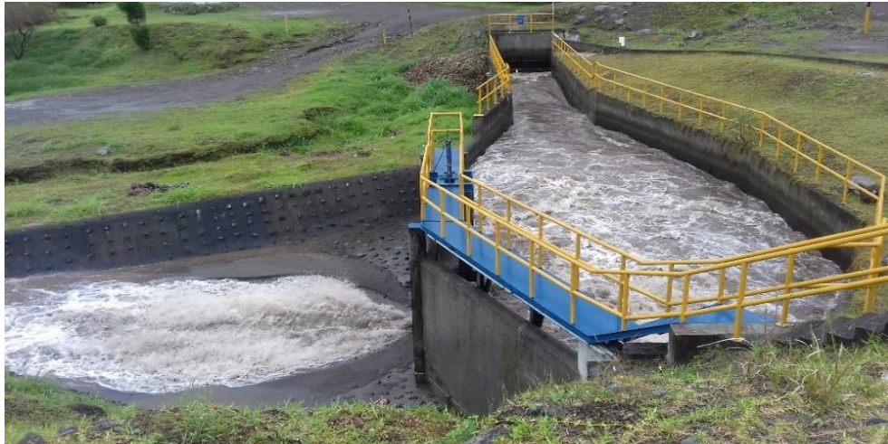
Figure 5-1 Shows the flow in Settling basin during rainy season.
