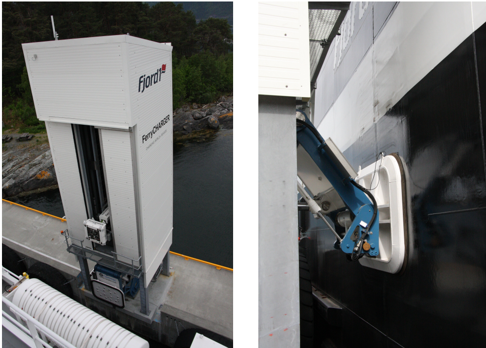
Figure 4.2: The charging tower "FerryCharger" and automated docking solution at the Anda-Lote site. Source: Teknisk Ukeblad
