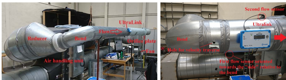
Figure 1 Left: Picture of the lab setup for testing Lindab UltraLink and VelociCalc 8388 and compare with calculated airflow rates found with the orifice plate. Right: setup used for the presented measurement results.
