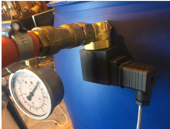
Figure 9.17: Solenoid Valve installed on the tank
