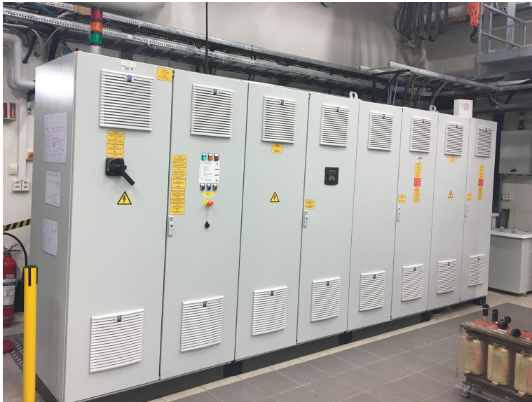
Figure 7.2: 200kVA Controlled Voltage Source
