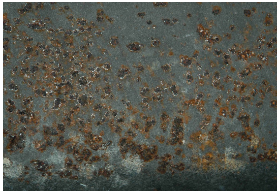
Figure 7: Example of pitting corrosion on steel, with the characteristic local pits or holes in the surface [16].
