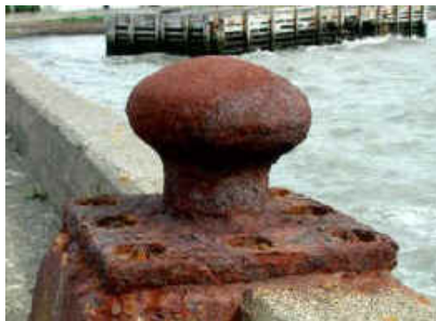
Figure 5: A typical uniform corrosion damage where the damage is evenly distributed over the surface [14].
