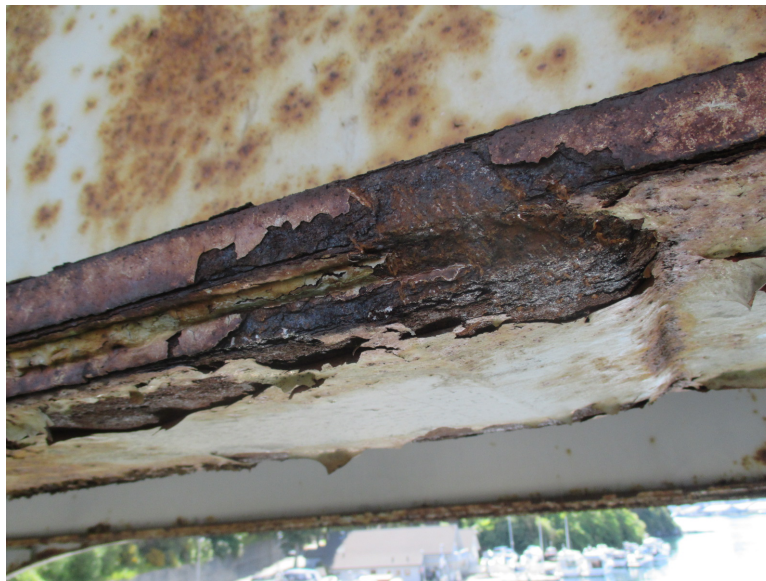
Figure 13: Illustration of corrosion on the steel construction of a bridge. This type of corrosion damages is often referred to as “red rust” because of the characteristic reddish colour. The image is downloaded from Brutus management system [21].
