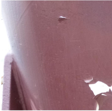
(a) Paint flaking classified as Red corrosion, steel construction by all networks 6-9.
