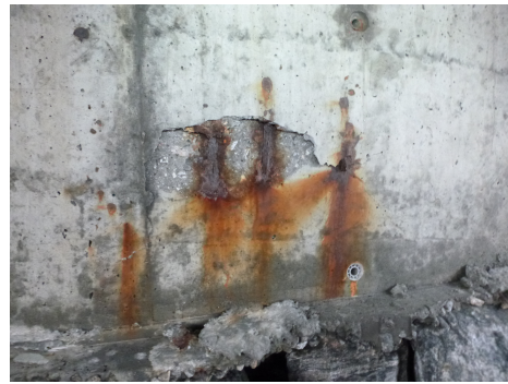
(b) Red corrosion, rebar classified as Red corrosion, steel construction by networks 2-9.
