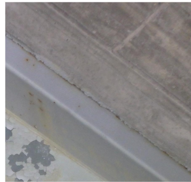
(d) Paint flaking classified as Red corrosion, steel construction by networks 6, 7 and 8, and as Red corrosion, rebar by network 9.
