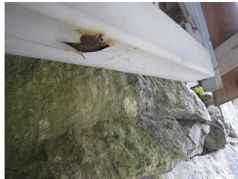
(d) Red corrosion, steel construction classified as Red corrosion, rebar by networks 2,3,5,6,7 and 9.
