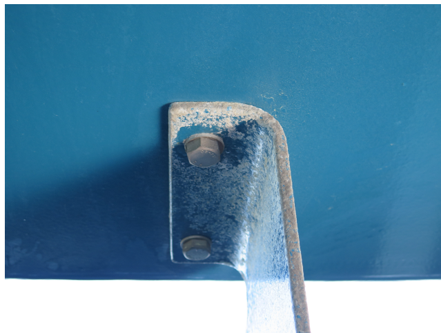
Figure 15: Illustration of corrosion on the steel construction of a bridge. This type of corrosion damages is often referred to as “white rust” because of the characteristic white-like colour. The image is downloaded from Brutus management system [21].
