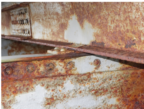
(e) Red corrosion, steel construction classified as Not corrosion by all networks, except network 6 (paint flaking).
