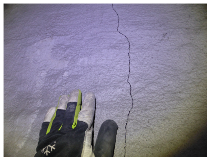
FIG. 6: Example of an image of not corrosion wrongly classified as red corrosion , rebar by networks 3, 4, 5, 8 and 9.
