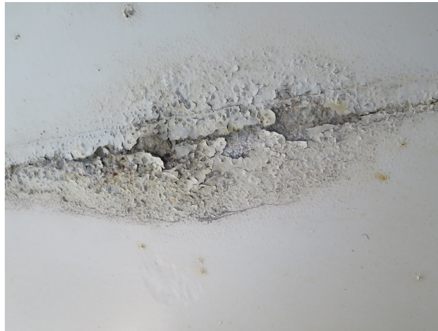
Figure 14: Illustration of corrosion on the steel construction of a bridge. This type of corrosion damages is often referred to as “white rust” because of the characteristic white-like colour. The image is downloaded from Brutus management system [21].
