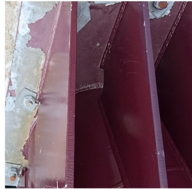
(b) Paint flaking classified as Not corrosion by networks 7, 8 and 9. Correctly classified as Paint flaking by network 6.
