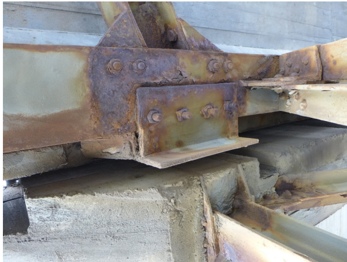
Figure 12: Illustration of corrosion on the steel construction of a bridge. This type of corrosion damages is often referred to as “red rust” because of the characteristic reddish colour. The image is downloaded from Brutus management system [21].
