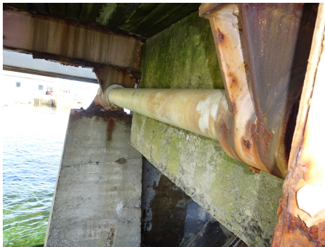
(c) Red corrosion, steel construction classified as Red corrosion, rebar by all networks 2-9.
