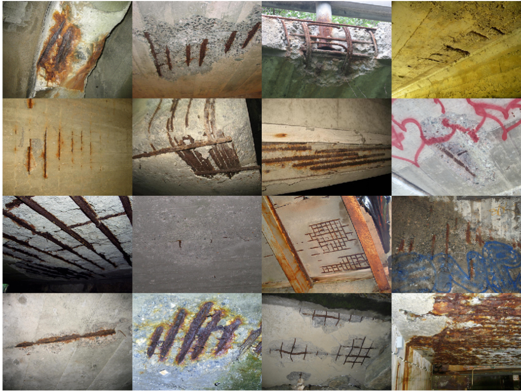
Figure 48: Examples of images collected in the class red corrosion, rebar .
