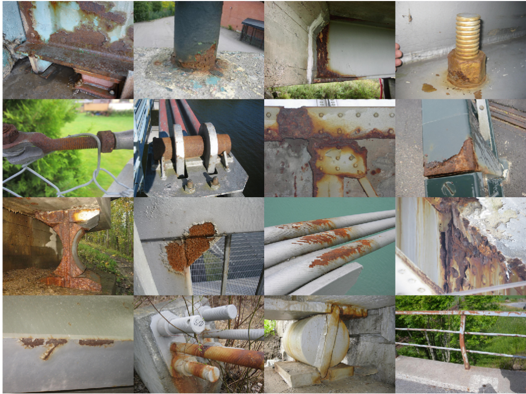
Figure 47: Examples of images collected in the class red corrosion, steel construction .
