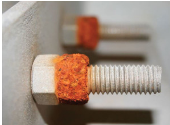
Figure 11: Galvanic corrosion on fasteners of carbon steel used on bolts of stainless steel [20]. In this case, one can compare with the overview in figure 10 and see that cast iron and steel in general are more anodic than stainless steel (316 and 304), and therefore the carbon steel fasteners are more exposed to corrosion than the bolts of stainless steel.
