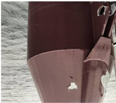
(c) Paint flaking classified as Not corrosion by networks 7, 8 and 9. The image was correctly classified as Paint flaking by network 6.
