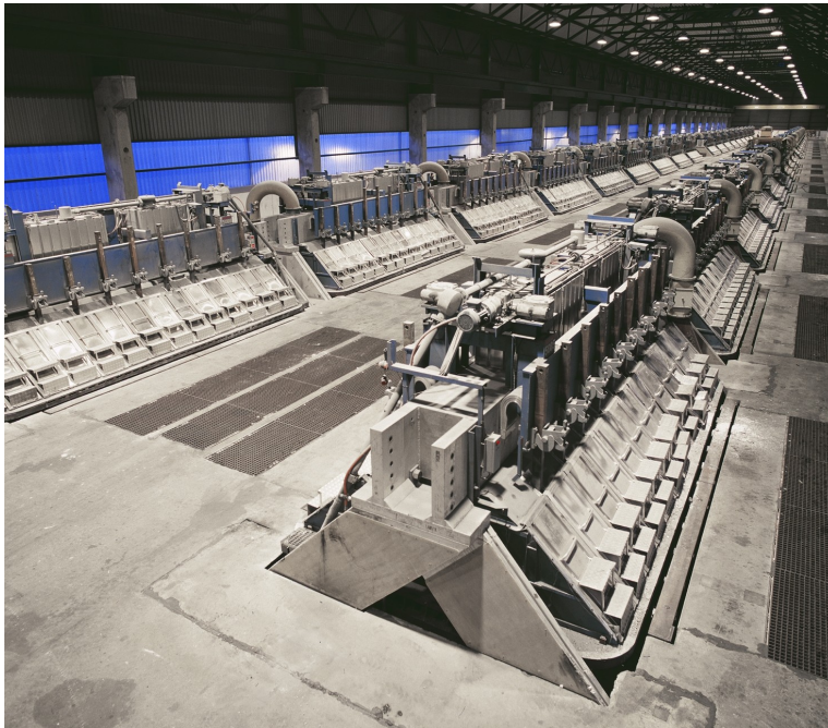
Figure 2.3: End-to-end potline at Alcoa Mosjøen (picture courtesy of Alcoa Mosjøen).
