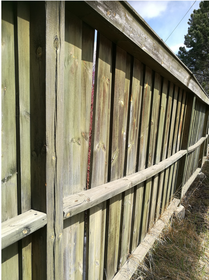
Figure 3.7: Wooden screen at Bekkestua, showing signs of decay and some leakages.
