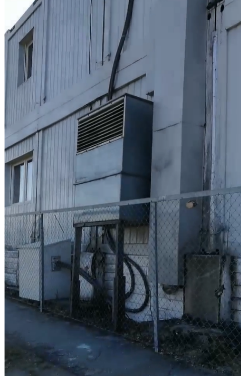
(b) Air condition system.
