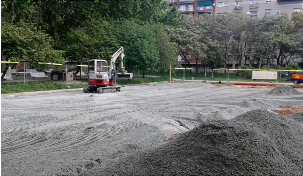
Figure 4.15: Application of an aggregate subbase layer in the basketball court (Civil Stone)
