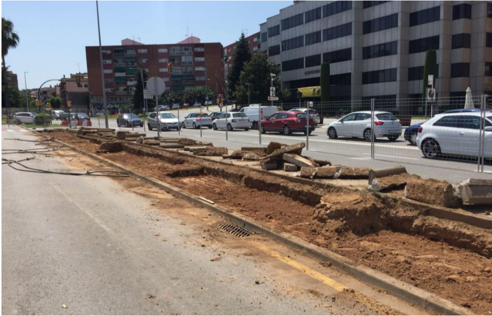
Figure 4.25: Demolition tasks in the existing median strip of the road (Civil Stone)
