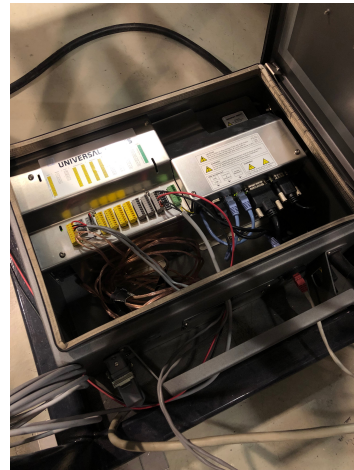
(b) The electrical interface.
