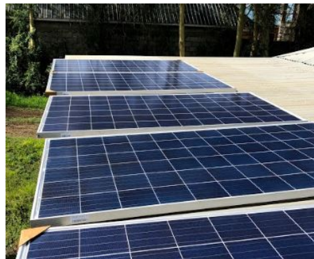
Figure 18: PV panels placed on the roof of the workshop rated 304.1 W and 36.2 V
