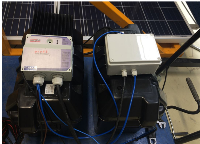
Figure 63: Battery setup with controller and fuse box
