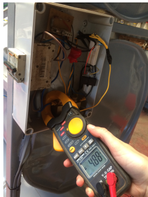
Figure 22: Measuring the current delivered from the PV panels on the roof
