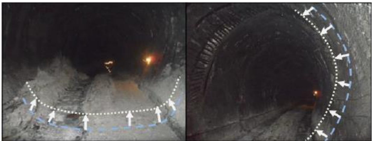
Figure 2-17 Squeezing in headrace tunnel of CHEP: Floor heave (left) and wall closure (right) (Basnet 2013)
