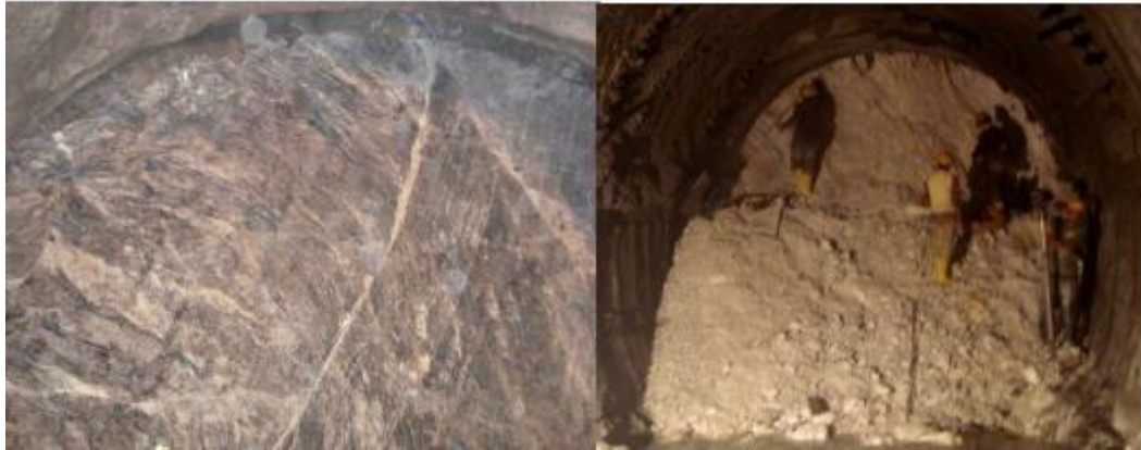
Figure 2-16 Rock mass condition at different chainage along headrace tunnel of Chameliya Hydroelectric Project (Basnet 2013)
